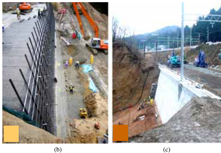
Fig. 17 (a) Railway embankment that collapsed during the 2004 Niigata-ken Chuetsu Earthquake and its reconstruction to a GRW RW having a FHR facing; (b) the wall during reconstruction; and (c) the completed wall (Morishima et al. , 2005)
