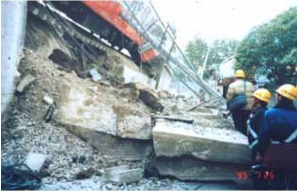
Fig. 14 Gravity type RW without a pile foundation at Ishiyagawa that collapsed during the 1995 Kobe Earthquake (Tatsuoka et al. , 1997, 1998)
