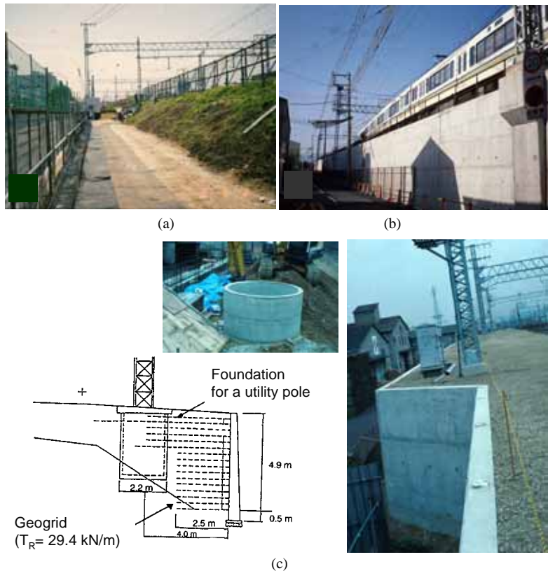
Fig. 10 (a) During; and (b) after reconstruction of embankment slope to GRS RWs having a FHR facing; and (c) a foundation for a utility pole constructed inside the geogrid-reinforced backfill; a rapid transit between Osaka and Kobe; average wall height = 5 m; total length = 1,300 m; and construction period = 1991 ~ 1992 (Tatsuoka et al. , 1997)
