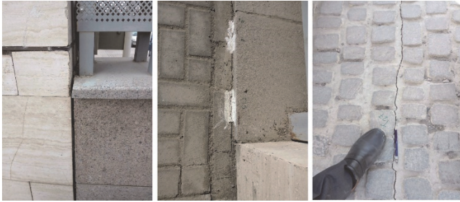
Fig. 3 Propagated cracks in the vicinity of the site after 24 m of excavation
